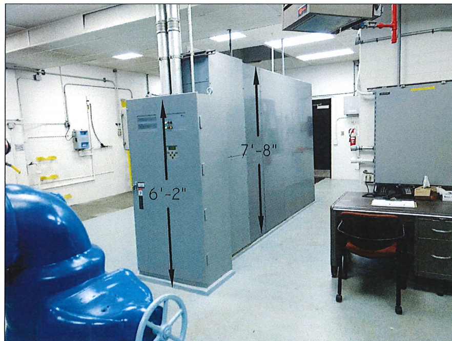
ELECTRICAL CABINET TOWARD DEEP WELL (OBSCURED)
