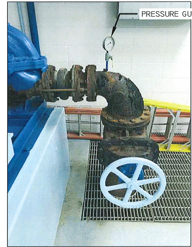
BOOSTER PUMP #1 SUCTION PIPE
