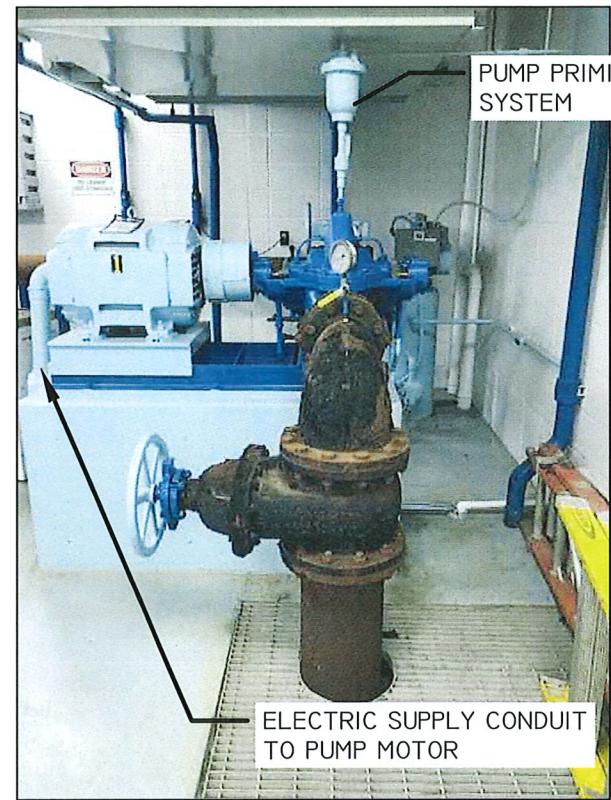
BOOSTER PUMP #1 SIDE VIEW
