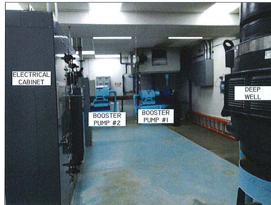
ELECTRICAL CABINET FROM ACCESS DOOR.
