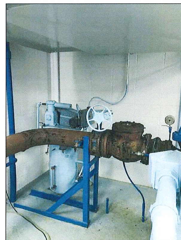
BOOSTER PUMP #1 DISCHARGE PIPE
