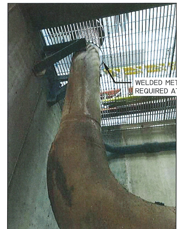
PIPE OPENING THROUGH GRATING
