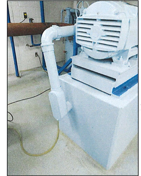
ELECTRIC SUPPLY CONDUIT
